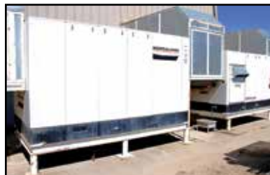
VIEW OF COMPRESSORS
