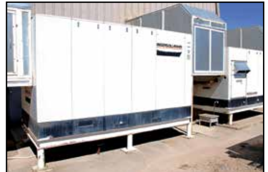
VIEW OF COMPRESSORS
