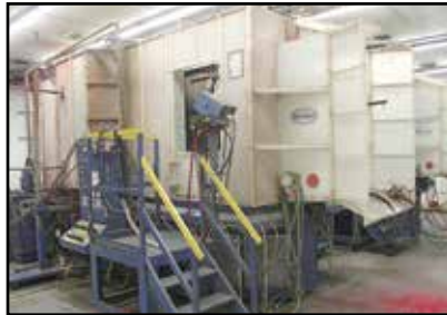
NORDSON PAINT BOOTHS
